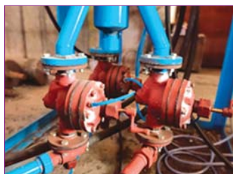
Pneumatic Grit Valve
